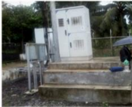
Legacy BTS equipment and rectifier system
