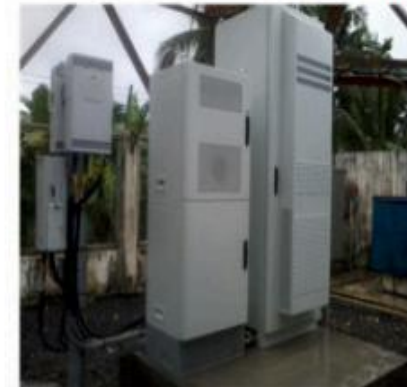
From legacy outdoor BTS equipment and rectifier system to new outdoor set-up using IP 55 cabinets, high efficiency rectifier system with 5 hour battery back up time
