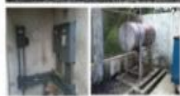
End of Useful Life Genset, Change Over Switch and fuel tank with no remote monitoring capability
