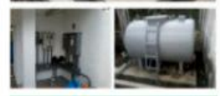
New Genset, Change-over Switch and Fuel Tank with intelligent remote monitoring system
